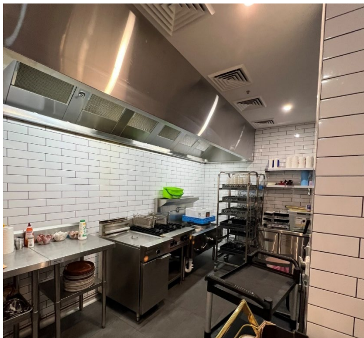
Figure 40 Industrial kitchen at 94 Hay Street.
